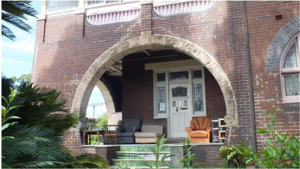
Figure 27 — No 17 Railway Terrace, showing details of stained glass windows, original stained glass front doors and side lights and verandah features. There is evidence of cracking of tiles in the stair treads (Source: NBRSPARTNERS, January 2015)
