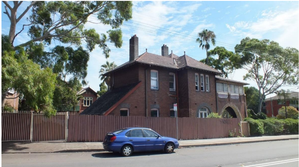
Figure 23 — No 17 Railway Terrace, North and East Elevations, taken from Railway Terrace, showing the slate roof, timber framed, double-hung sash windows with clear glass (Source: NBRS+PARTNERS, January 2015)
