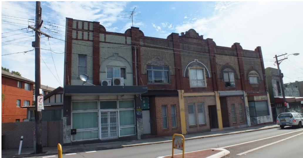
Figure 10 — Detail of Federation terrace group, located at Nos 21-29 Railway Terrace. The Federation terraces remain intact on the first floor and mostly modified shopfronts at ground level and awnings removed (Source: NBRSPARTNERS, January 2015)
