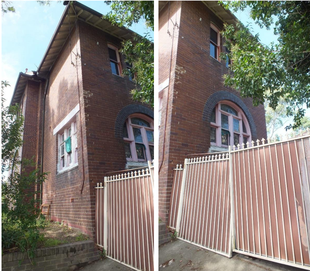
Figure 29 — No 17 Railway Terrace, South Elevation showing stained glass windows at ground level near driveway off Hunter Street. Later addition gates in poor condition (Source: NBRSPARTNERS, January 2015)
